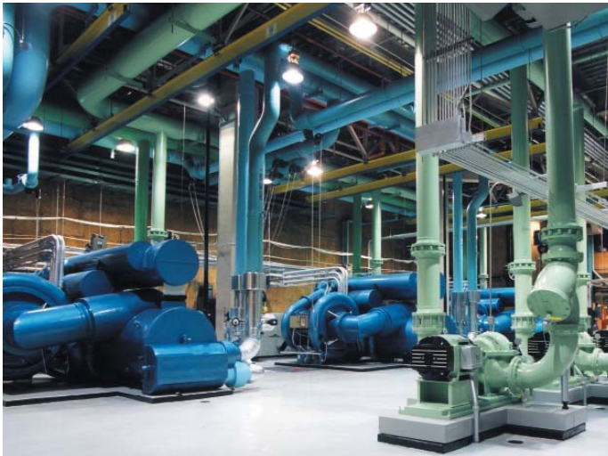
Marathon Oil Tower's central plant (pictured above) is the heart of building HVAC and electrical operations. A new, state-of-the-art Energy Management System, along with a full building lighting retrofit in 2007 will reduce electric consumption by more than 3 million KWH each year!
